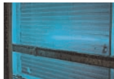
A large hospital air conditioning coil irradiated with UVC lights.
