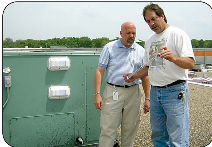
Bruce Strandberg (left) and Randy Remer prepare for annual changeout of the replaceable UVC Emitter™ tubes in the rooftop air handling units.
