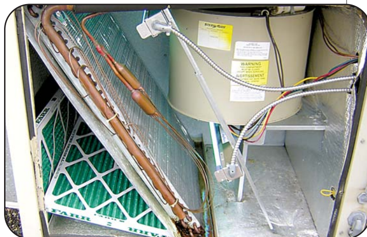
UVC Emitters™ in the air handling units have successfully eliminated both surface mold and airborne mold spores at Medicine Lake Properties.
